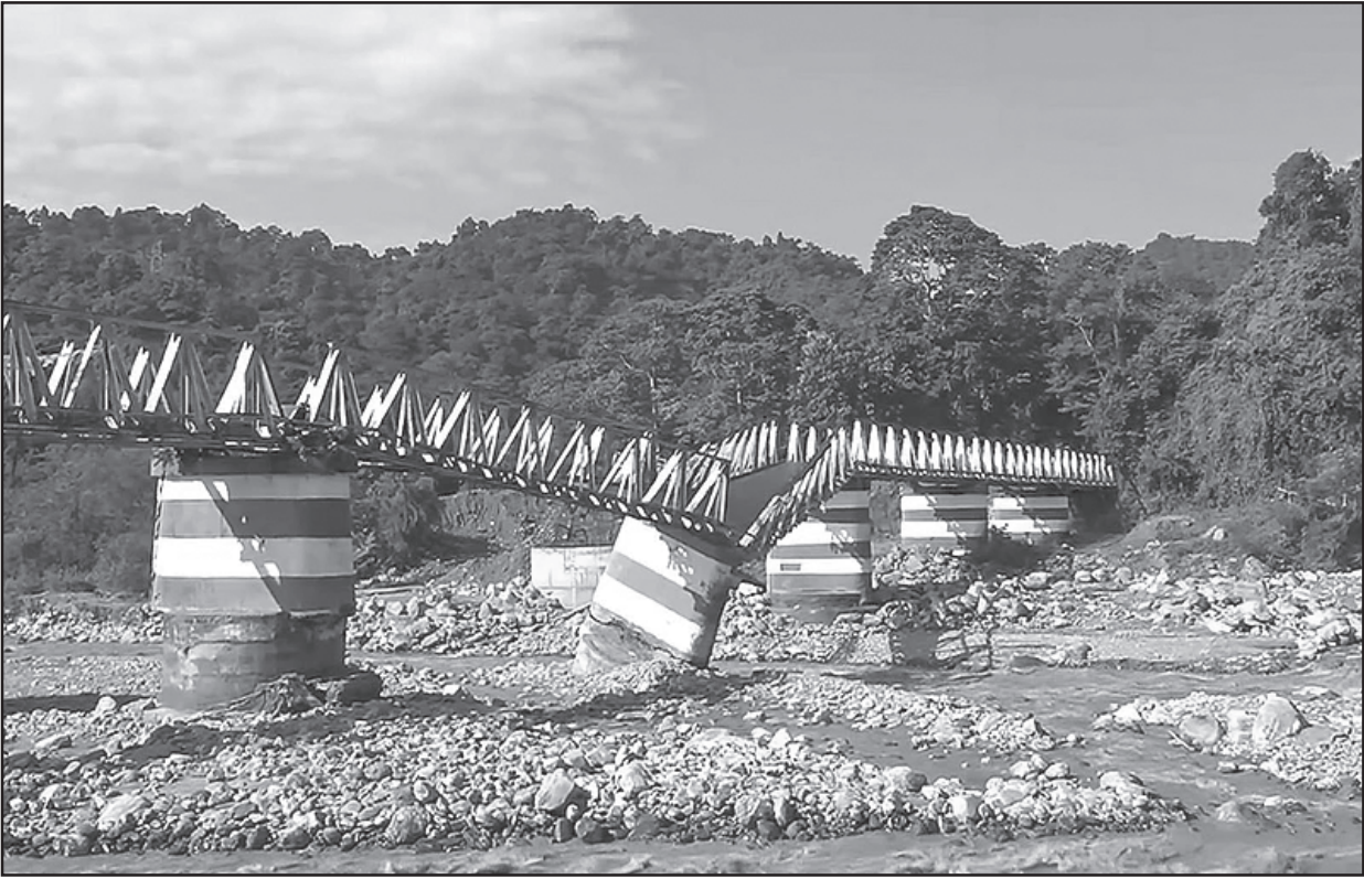
Damaged Dudhia iron bridge after landslides and heavy rainfall, in Darjeeling on Tuesday.
